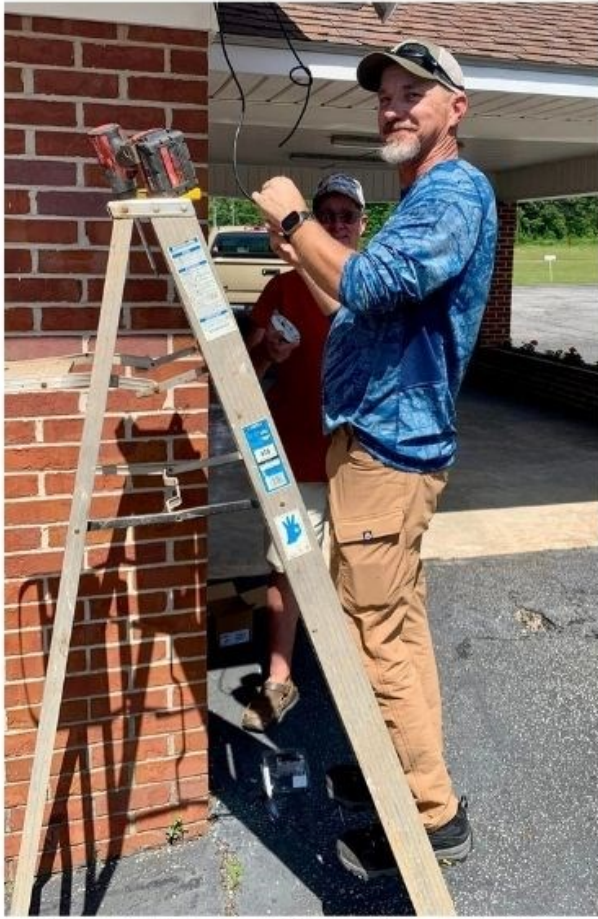
New Security Cameras are installed around the entire church.
